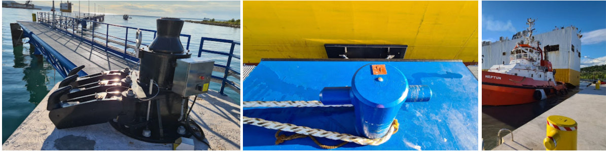
Figure 8: Mooring Hooks (PM), Bollards on mooring dolphins (1-5) and Shore bollards (6-9)
