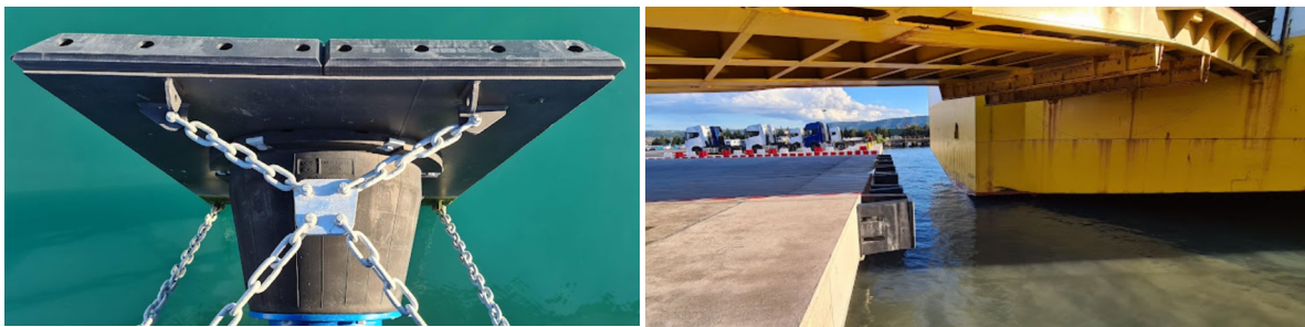
Figure 9: Fenders on mooring dolphins and fenders on access pier
