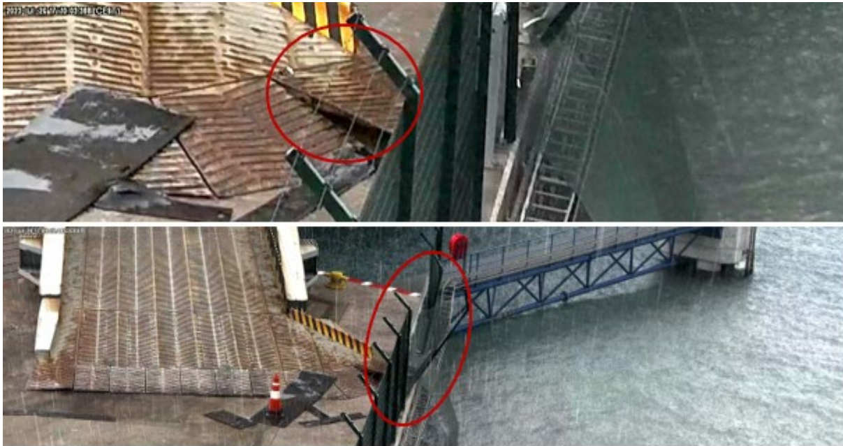
Figure 6: Damaged ramp flap and security fence (VNC)
