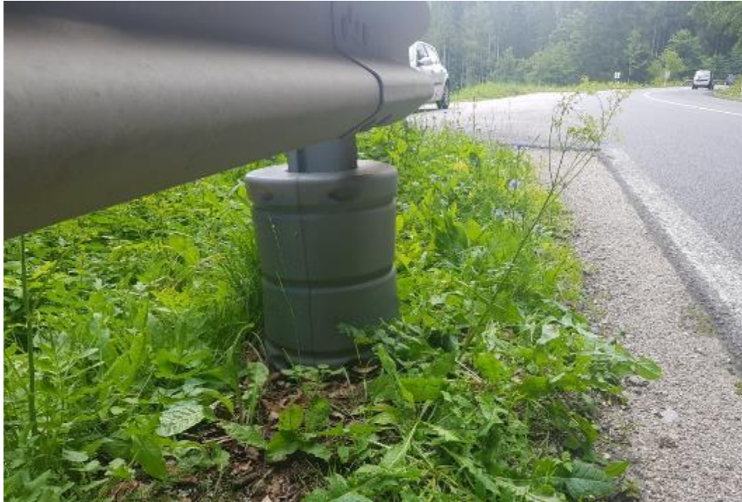
Figure 9: Properly installed MIP on a SGR post (source: B. Matko and U. Brumec).
