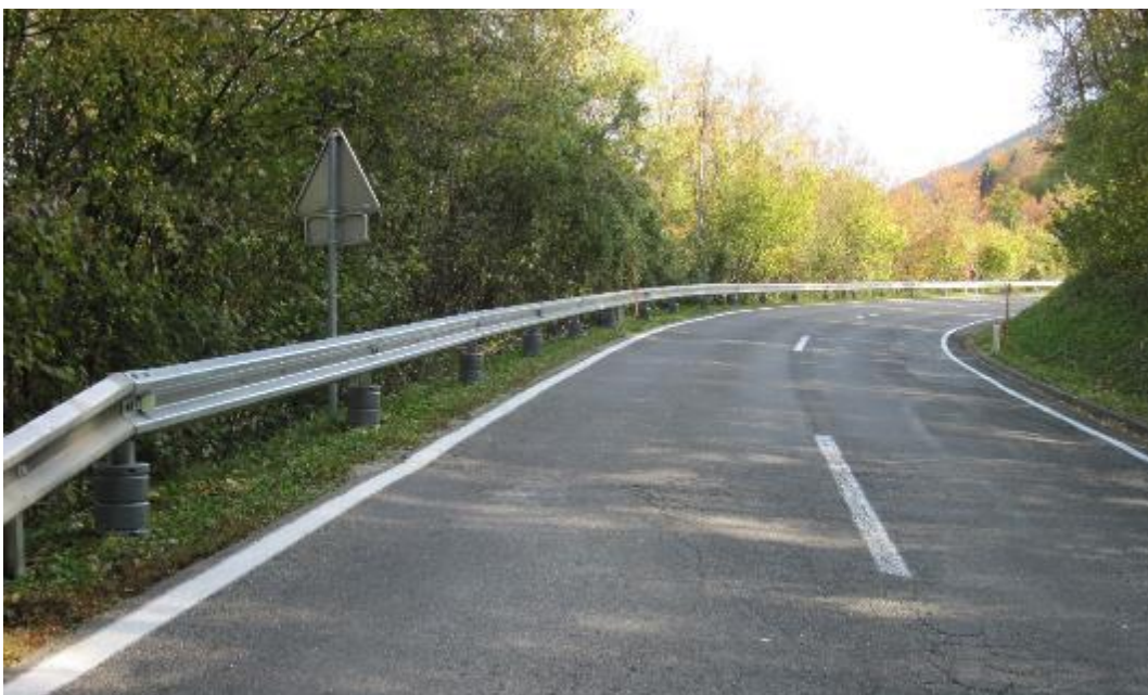
Figure 10: Properly installed MIP on a SGR post (source: B. Matko and U. Brumec).
