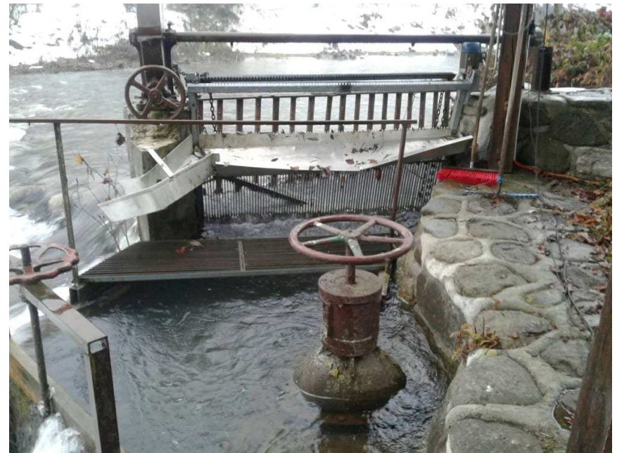
Photo 10 – valve and inlet of water to the fish farm
