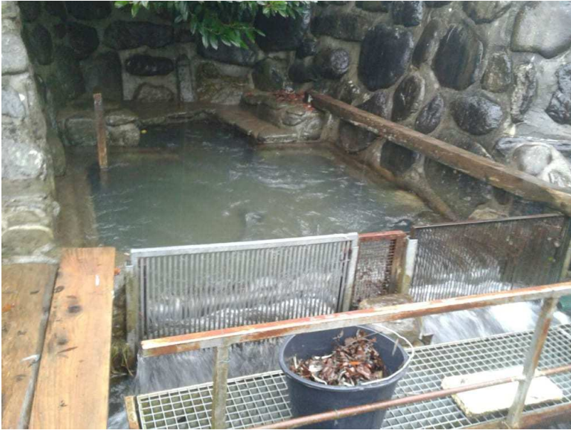
Photo 5 – cleaning grid at the inlet to the first concrete
